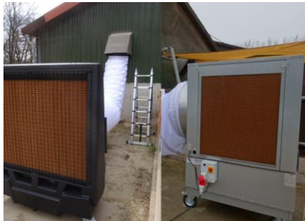
Evaporative cooling pads (above)
