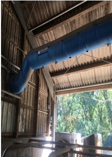
Ventilation and cooling tube with air outlet jets above a row of lying cubicles (right)
