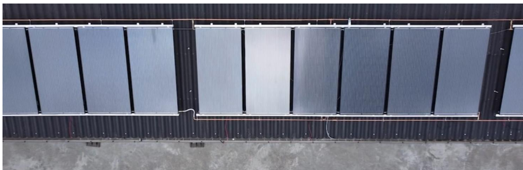
Figure 1: PVT collectors at ILVO swine farm in Belgium, before insulation of pipes
