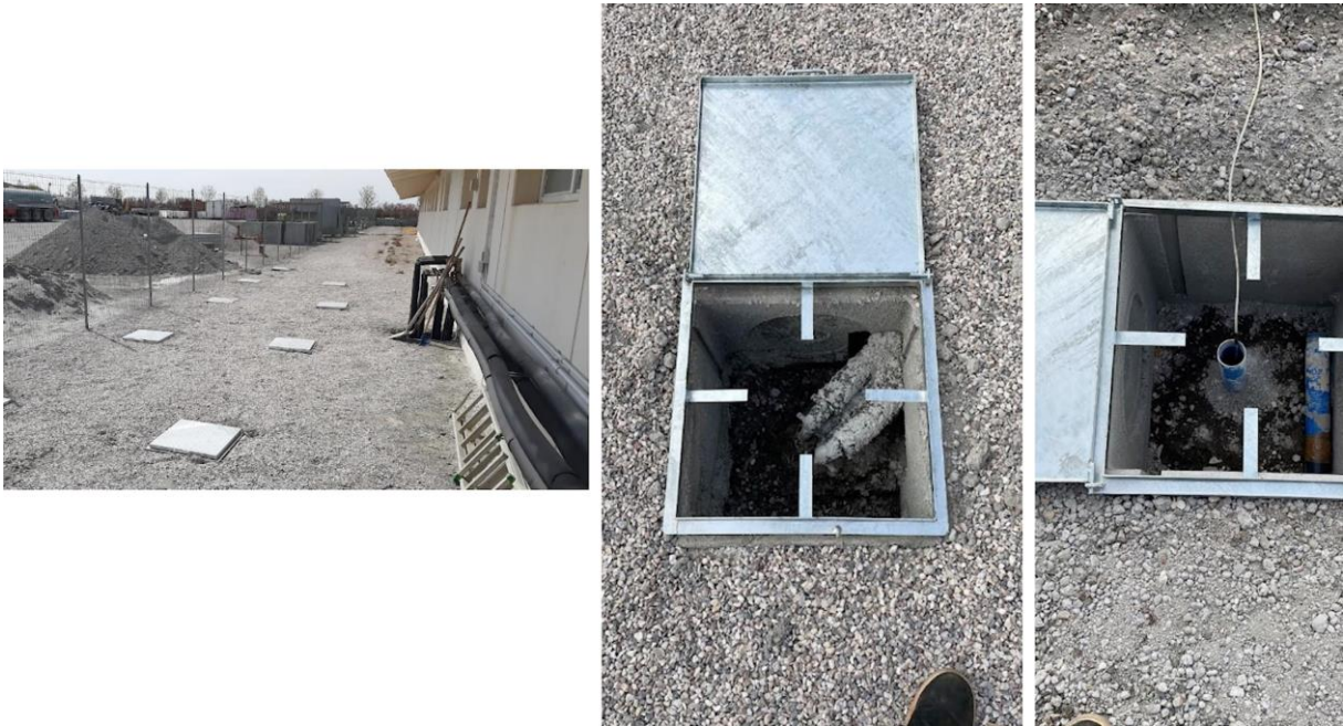
Figure 3. Snapshot from the RES4LIVE final video showing the geothermal energy storage installation at GOLINELLI swine farm, Italy.
