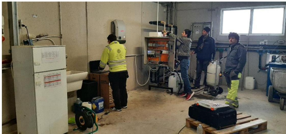
Figure 15. Installation and connections of the geothermal storage with the solar station.
