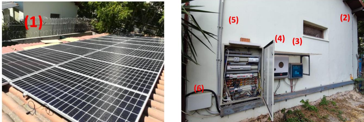
Figure 26. The PVs installed on the rooftop of a building nearby the AUA poultry farm (left) and the PV connections to the inverter and the electrical panels (right).
