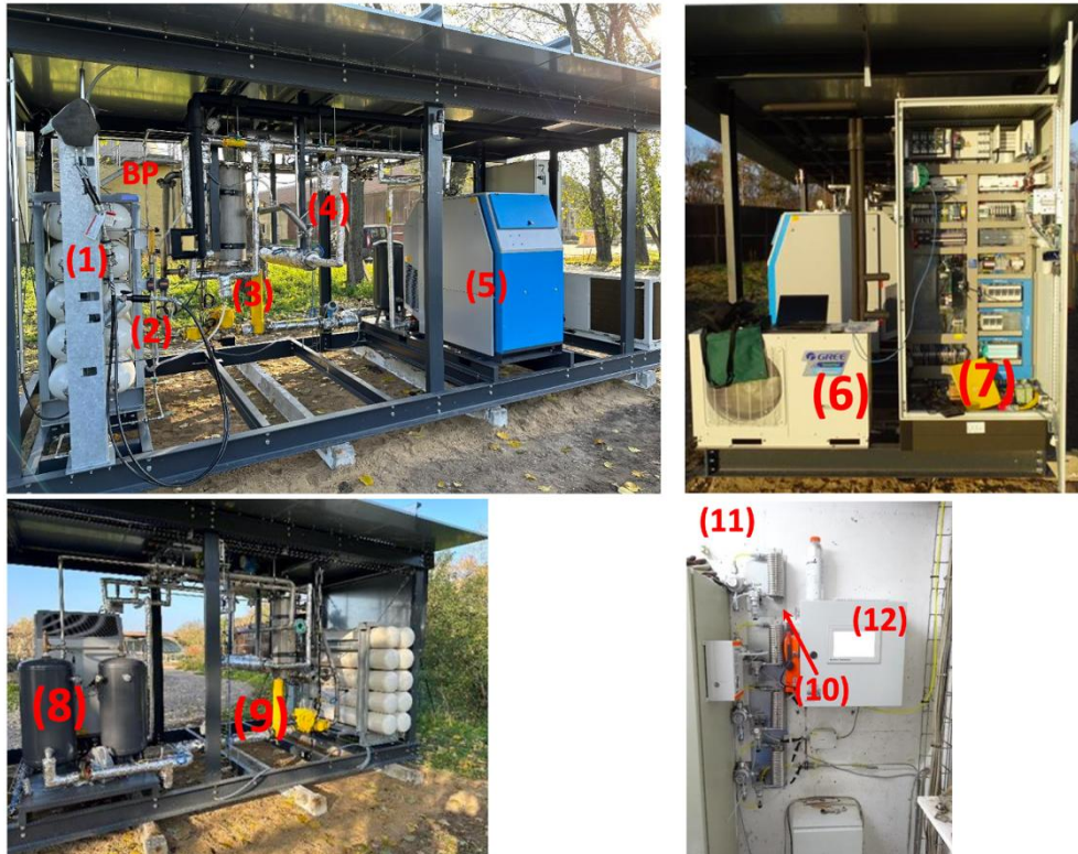
Figure 20. View of the CNG filling station with the biogas plant in the background (upper-left), side view (upper-right), rear view (lower-left) and gas component sensors (lower-right) of the biogas plant.
