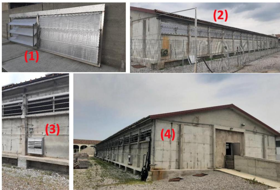
Figure 18. Detail of the new windows (1) – The building after the installation (2) – Windows after actuating opening (3) - West side of the hog barn with windows open (4).
