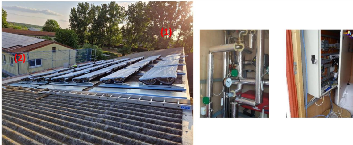
Figure 21. The installed PVT system on the LVAT barn rooftop (left) and the solar station with heat storage (right).
