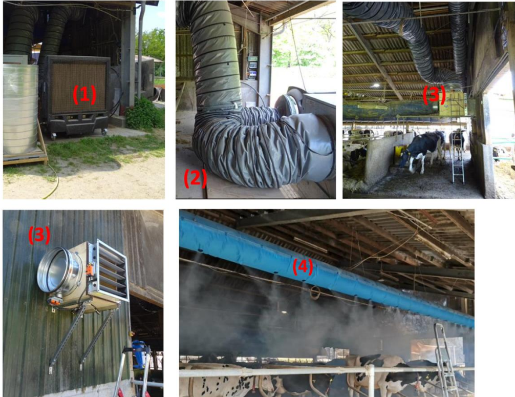
Figure 24. The evaporation cooler (upper-left), insulated influx tubes (upper-middle), bypass boxes inside (upper-right) and outside (lower-left) the welfare barn at LVAT, mixing ambient air with pre-cooled air and a entilation tube line above a single row of lying cubicles (lower-right).
