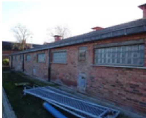
Figure 21: Picture of side external wall of fattening pig compartment at C1 case.
