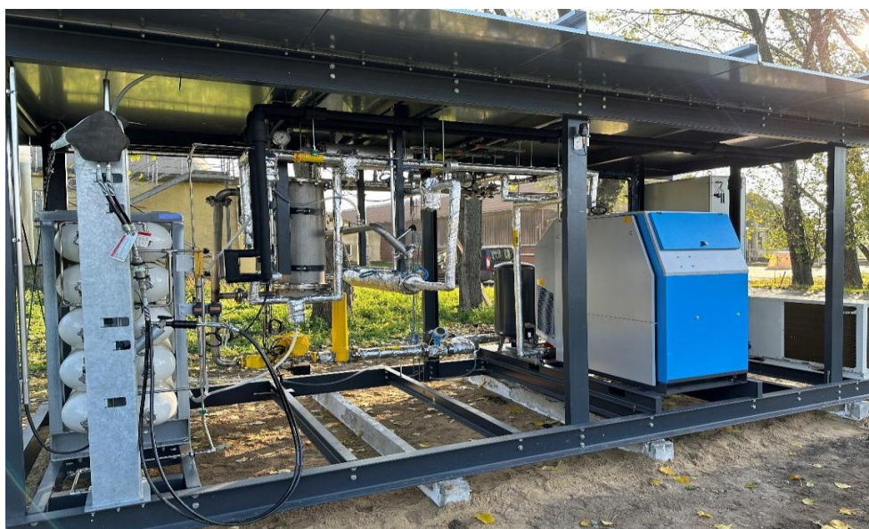
Figure 24. The biomethane upgrading and fuelling station.
