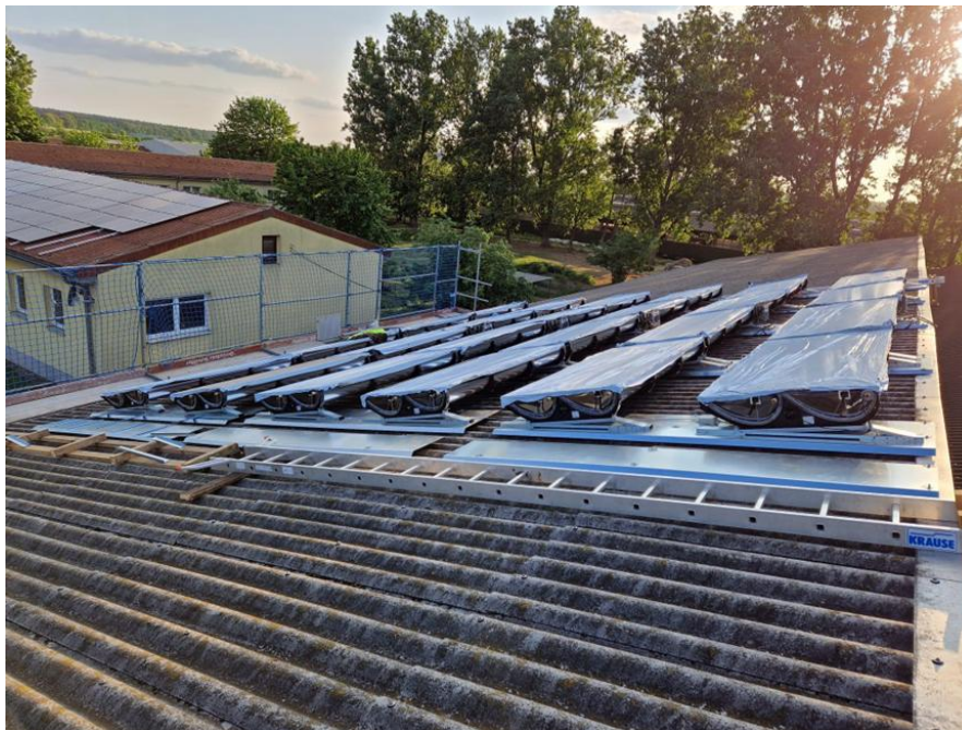
Figure 26. The PVT system at LVAT.
