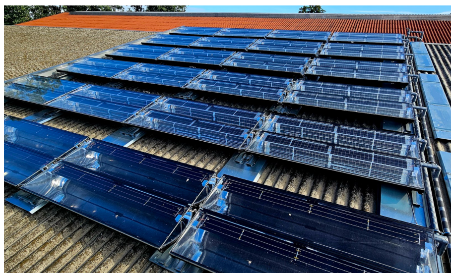
Figure 2: Concentrating PVT installation at LVAT dairy farm in Potsdam, Germany
