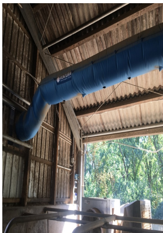
Ventilation and cooling tube with air outlet jets above a row of lying cubicles (right)
