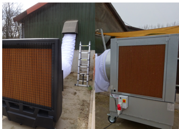
Evaporative cooling pads (above)
