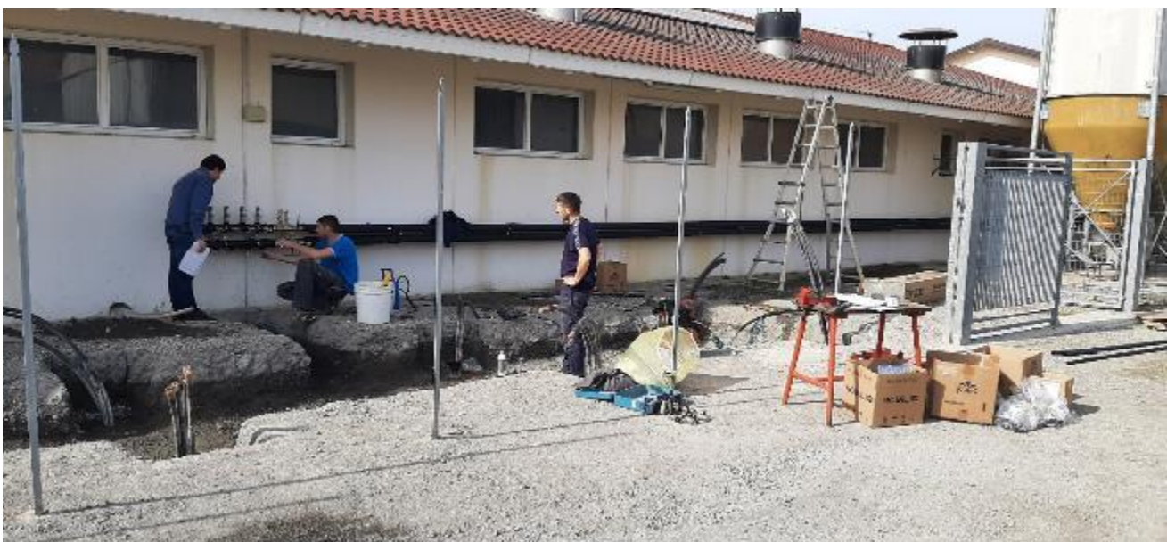
Supervision by UNIBO of RES4LIVE installations in Italian farm: Francesco Tinti is checking the collectors
